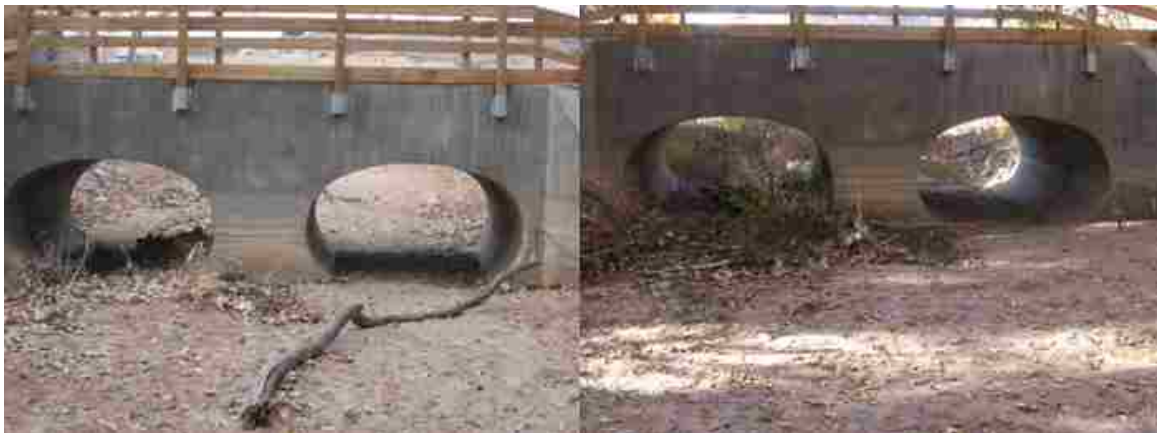
Figure 2-13: South Culvert Blockage Increased from 02/2010 (left) to 11/2010 (right)
