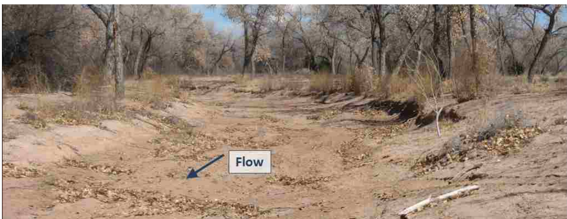
Figure 5-4: Bank Erosion along the Major Bend (02/2010)
