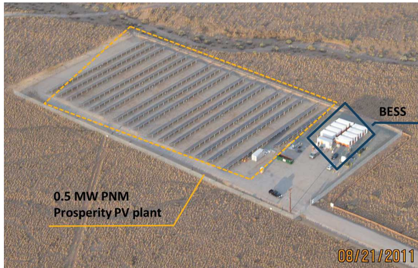
Figure 2.1: Aerial view of the 0.5 MW PNM Prosperity PV plant with battery storage
