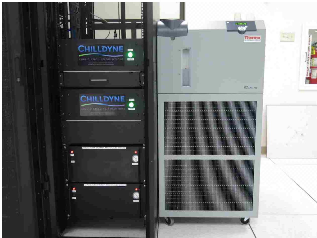
Figure 3: Image of the CDUs with vacuum pumps (left), and standalone chiller (right).
