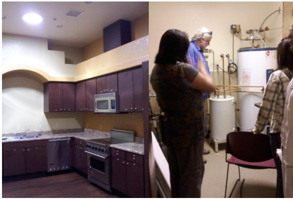
Figure 39. Hualapai Social Services Building features. Left: Solar light tubes provide lighting. Right: High efficiency water heater and fixtures. Source: Personal photo.
