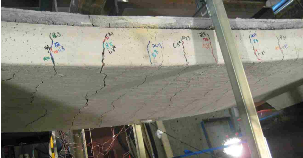
Figure 5.16: Flexural cracking of the strengthened concrete slab
