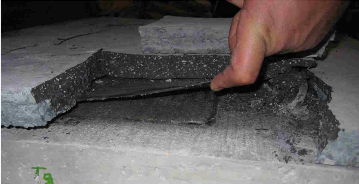
Figure 5.19: Debonding of the CFRP from the NVC substrate
