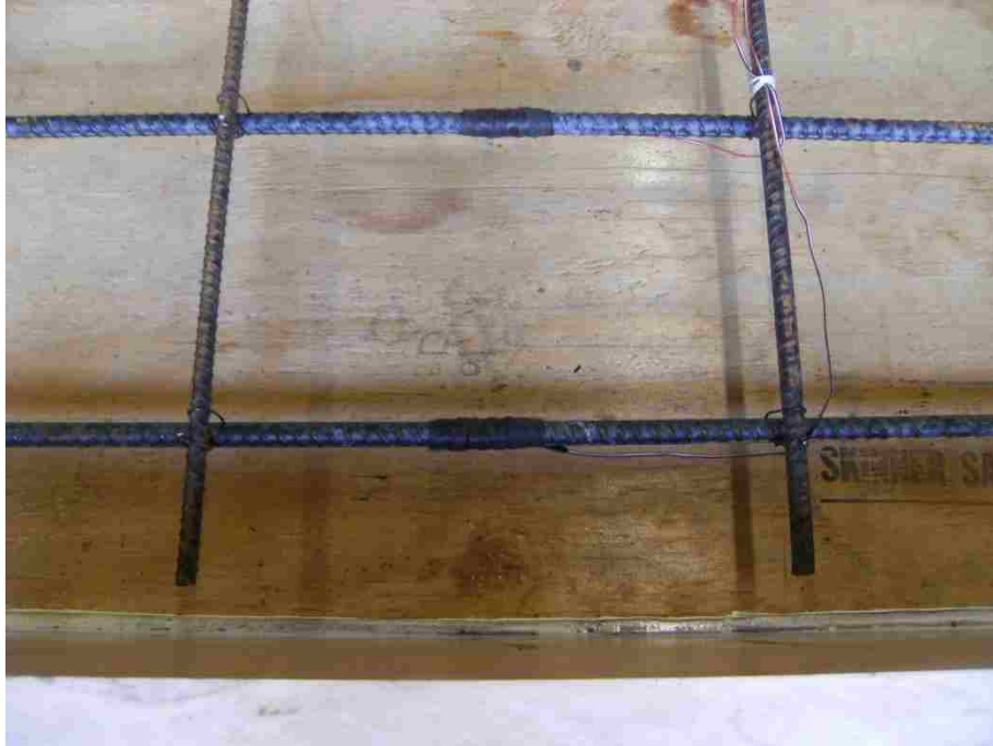
Figure 3.17: Embedded strain gauge protection
