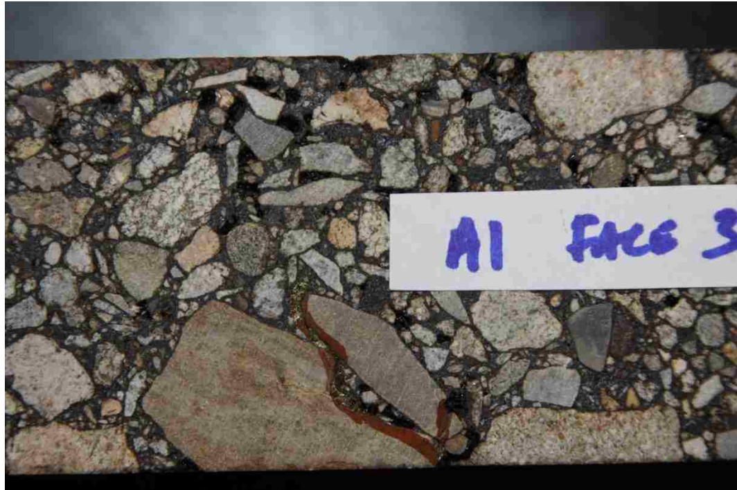
Figure 6.2 Fatigue Crack Propagating Upwards in HMA Beam Sample SP-II-A1
