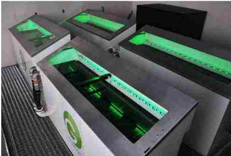
Figure 2.5. Immersion cooling - CGG Datacenter, Houston TX.
