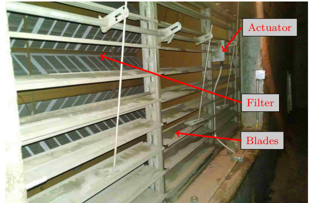
Figure 3.7: Outside air damper system that has a mechanical actuator controlled by the DDC.
