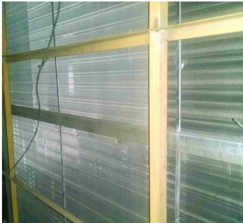
Figure 3.10: CHW cooling coils that transfer heat from the air to the water.
