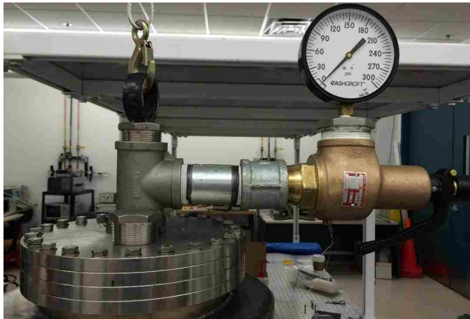
Figure 32: Relief Valves (150 psi) added to the Inner and Outer Chamber Inlets
