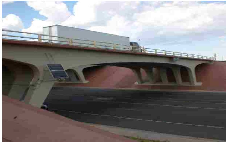
Figure 5-58 Solar power system installed on Bridge 7937 to provide clean renewable energy for the SHM system.
