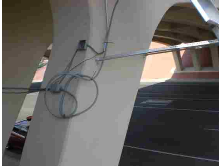
Figure 5-51 Electrical boxes and conduits to pass power to the SDA using the solar panels.
