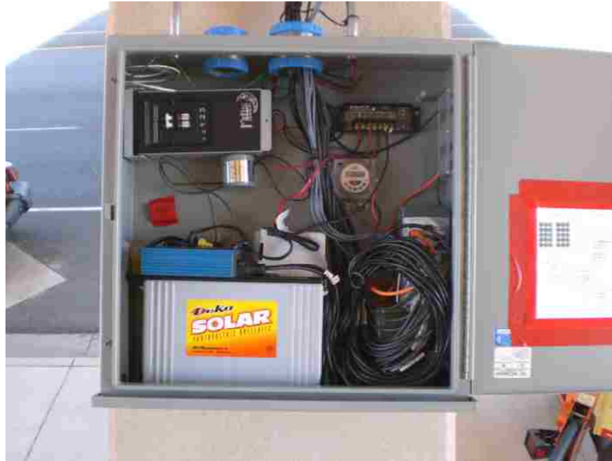
Figure 5-57 Data acquisition system, rechargeable batteries, power inverter, digital timer switch and the wireless modem located at the steel box.
