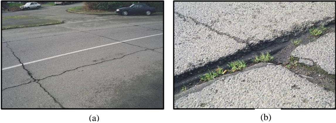
Figure 7. Reflection crack overview on flexible asphalt pavement (a), and reflection crack closeup (b) (From Miller & Bellinger, 2003).
