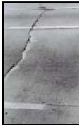
Figure 16. Faulted transverse joints on rigid concrete pavement (From Miller & Bellinger, 2003).
