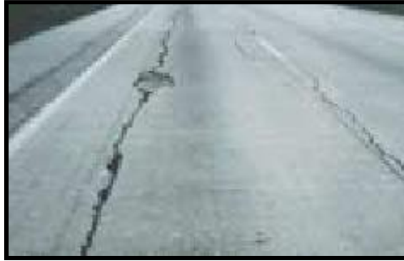
Figure 13. Longitudinal cracks on rigid concrete pavement (From Miller & Bellinger, 2003).
