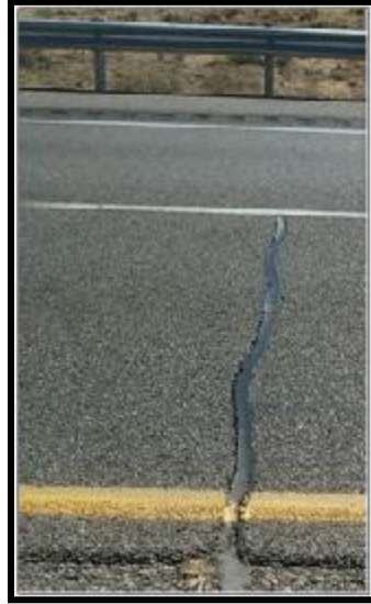
Figure 5. Sealed transverse crack on flexible pavement (From Miller & Bellinger, 2003).
