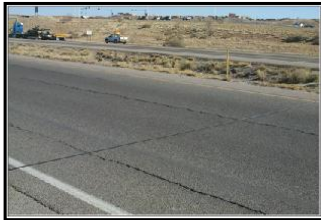
Figure 4. Longitudinal cracks on flexible asphalt pavement (from Miller & Bellinger, 2003).
