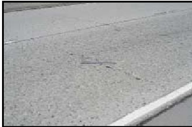
Figure 14. Transverse crack on rigid concrete pavement (From Miller & Bellinger, 2003).
