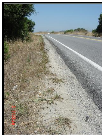
Figure 12. Lane-shoulder drop-off (From Miller & Bellinger, 2003).
