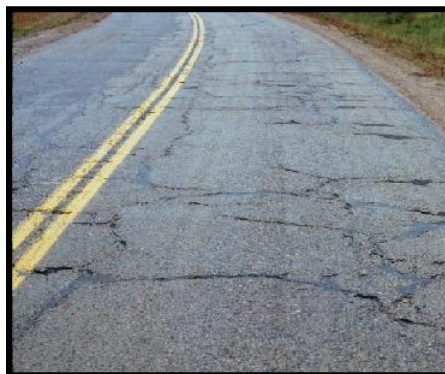
Figure 6. Block cracks on flexible asphalt pavement (From Miller & Bellinger, 2003).
