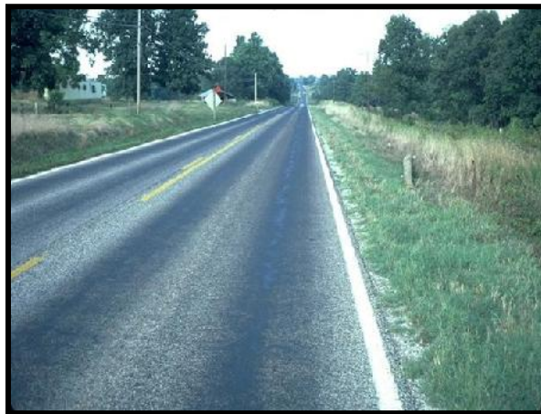
Figure 10. Bleeding on flexible asphalt pavement (From Miller & Bellinger, 2003).
