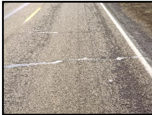
Figure 11. Raveling on flexible asphalt pavement (From Miller & Bellinger, 2003).
