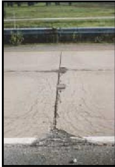
Figure 15. Durability cracking on rigid concrete pavement (From Miller & Bellinger, 2003).
