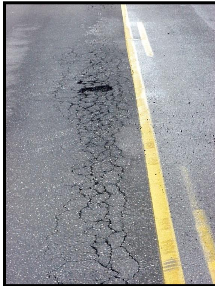
Figure 8. Pothole on flexible asphalt pavement (From Miller & Bellinger, 2003).
