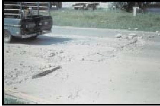
Figure 17. Severe blowups on a rigid concrete road (From Miller & Bellinger, 2003).
