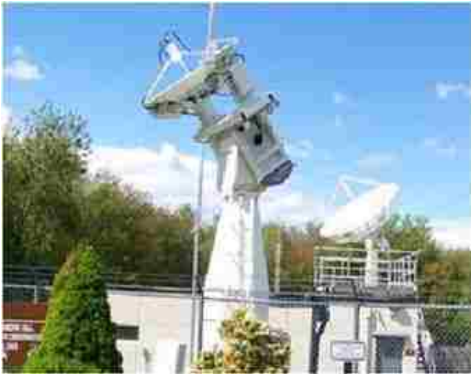
Figure 5: RSTN installation antennas.
