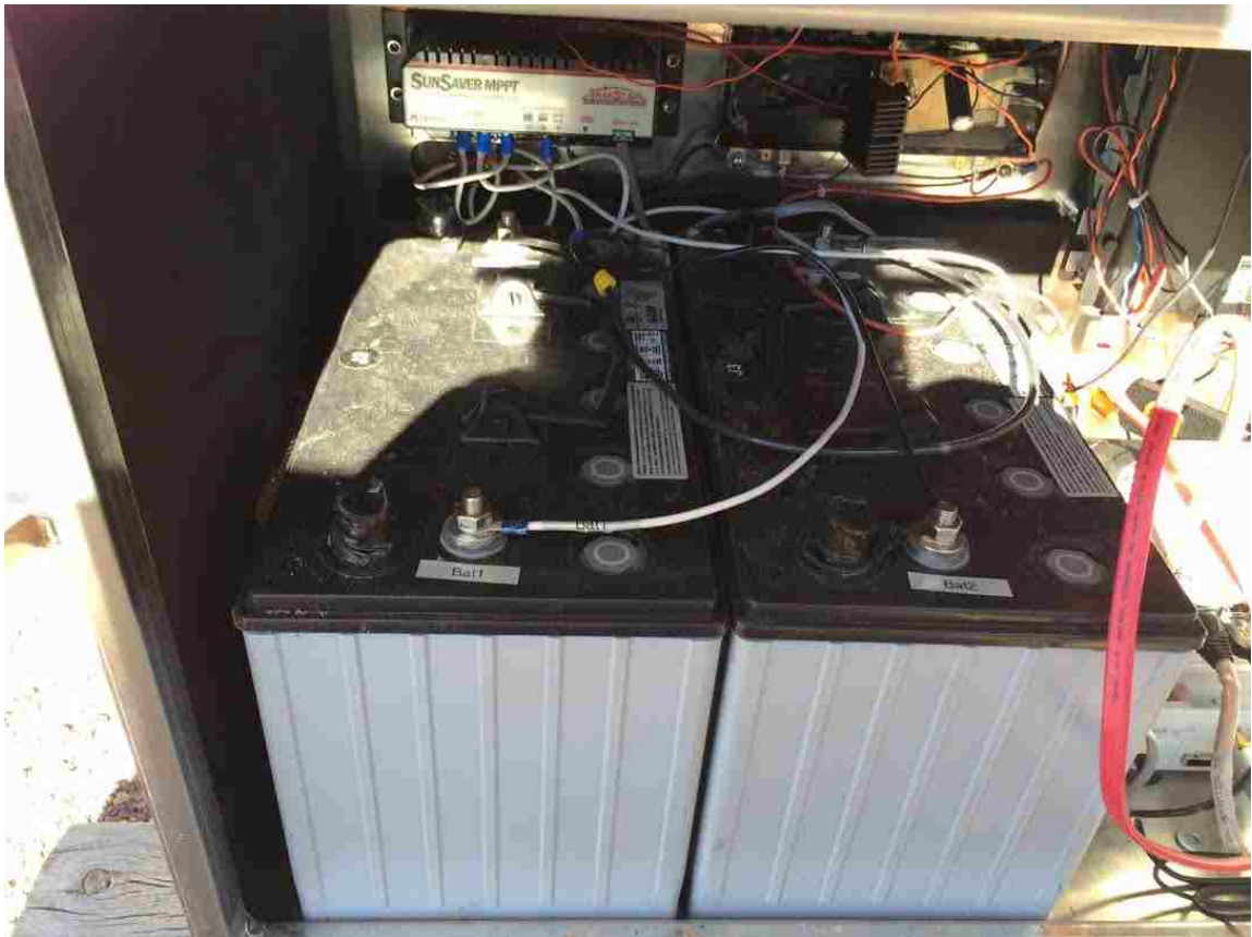
Figure 3.5: Showing charge controller, batteries, and voltage regulator for final stage amplifier, atop the tri-voltage SMPS block.
