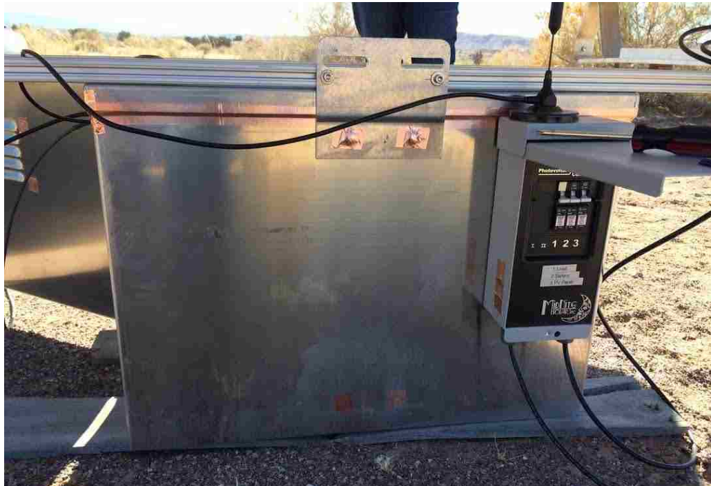
(b) Showing breaker box, cellular antenna, and PV power inputs.
