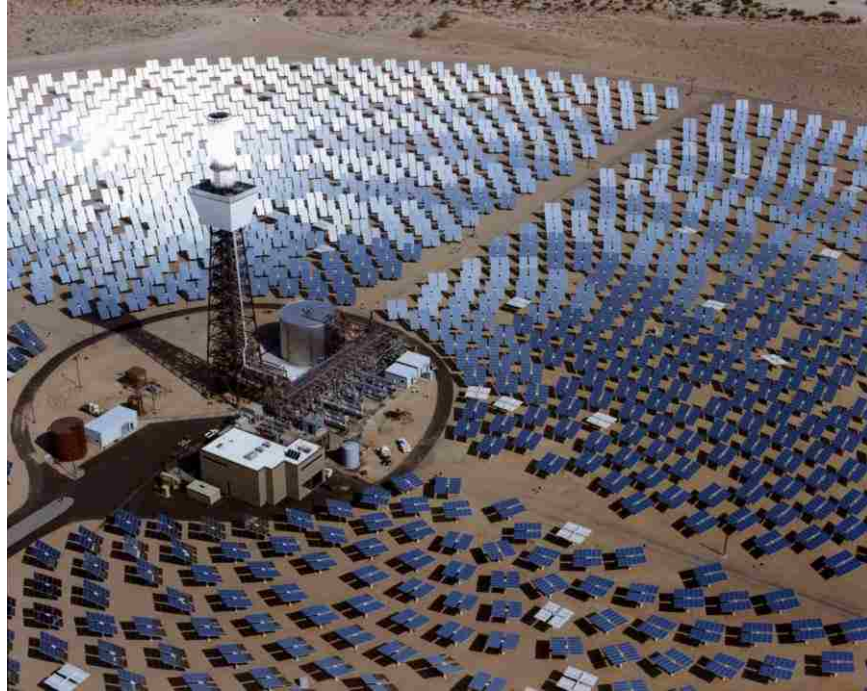
Figure 4. Solar Two 10 MWe CSP plant with central receiver tower and 1818 heliostats.
