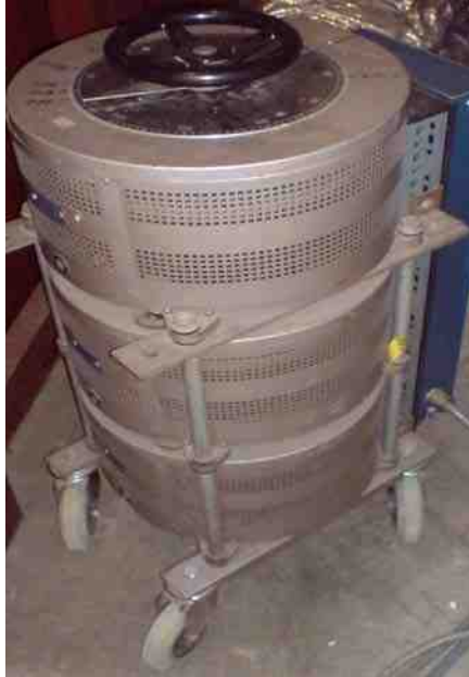
Figure 6.2d A three phase electrical transformer.
