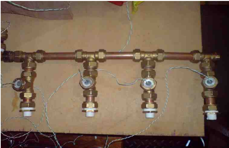
Figure 6.3a Manifold with thermocouples attached formed with compression fittings.
