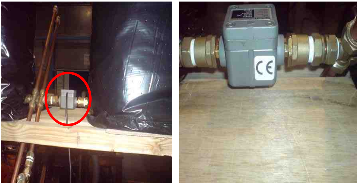
Figure 6.4g Mass Flow meter.
