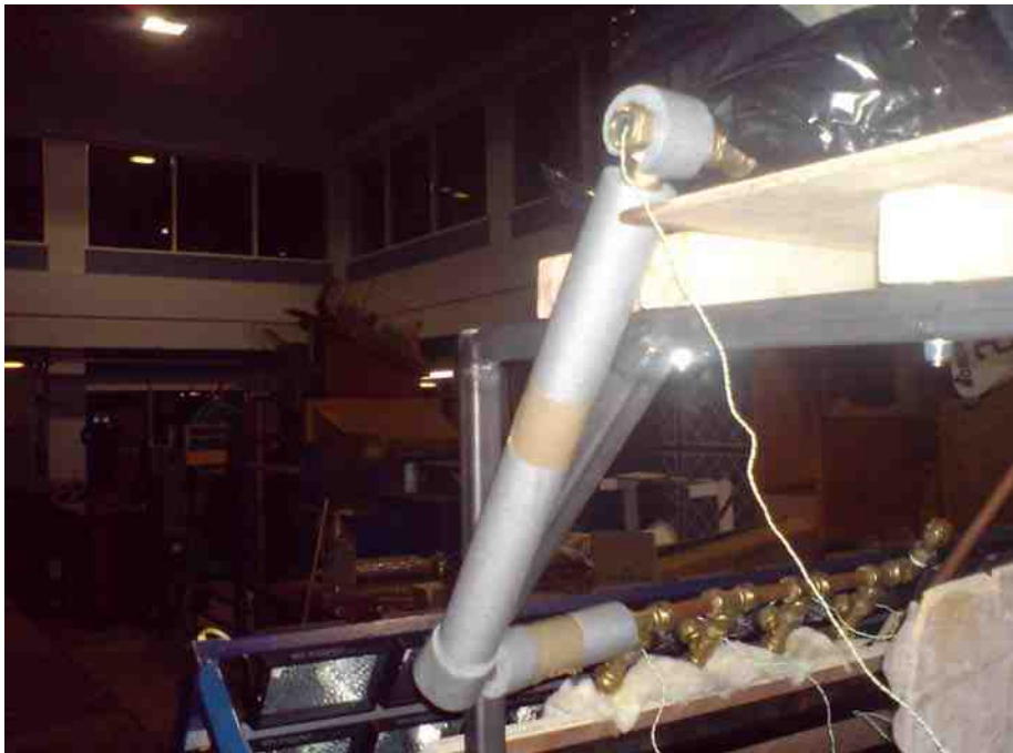
Figure 6.4c Insulated water tanks and copper pipes.
