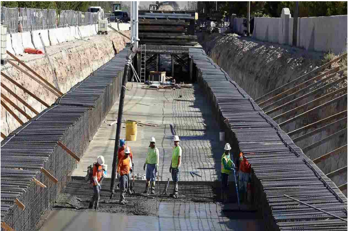
Figure 11. Workers building an underground storm drain in Northwest Las Vegas. (image courtesy of CCRFCD)
