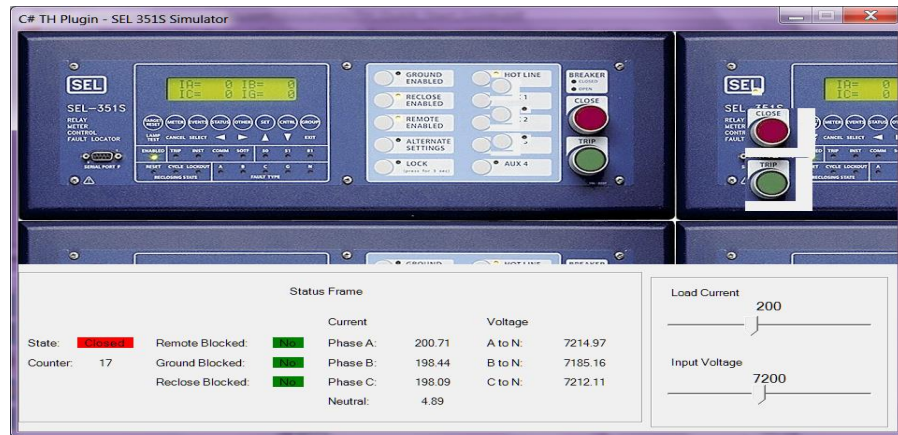
Figure 3.3 RTU displaying normal current flow
