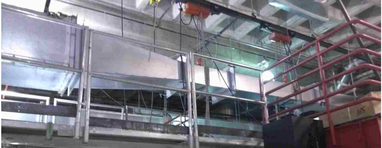
Figure 5.3: 12x18 Duct Test Setup
