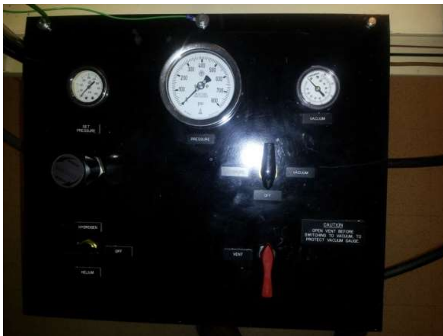
Figure 2.18 Gas Handling Unit
