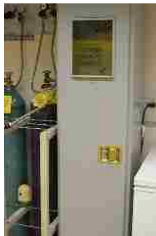
Figure 2.9: Gas cylinder storage
