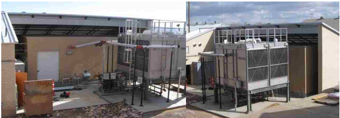
Figure 24. HVAC Central Chiller Plant and Cooling Towers.
