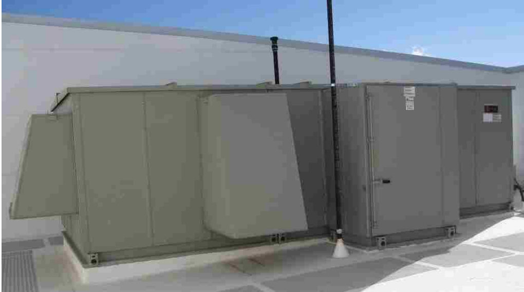
Figure 32. AHU-1 Roof-Top Installation.
