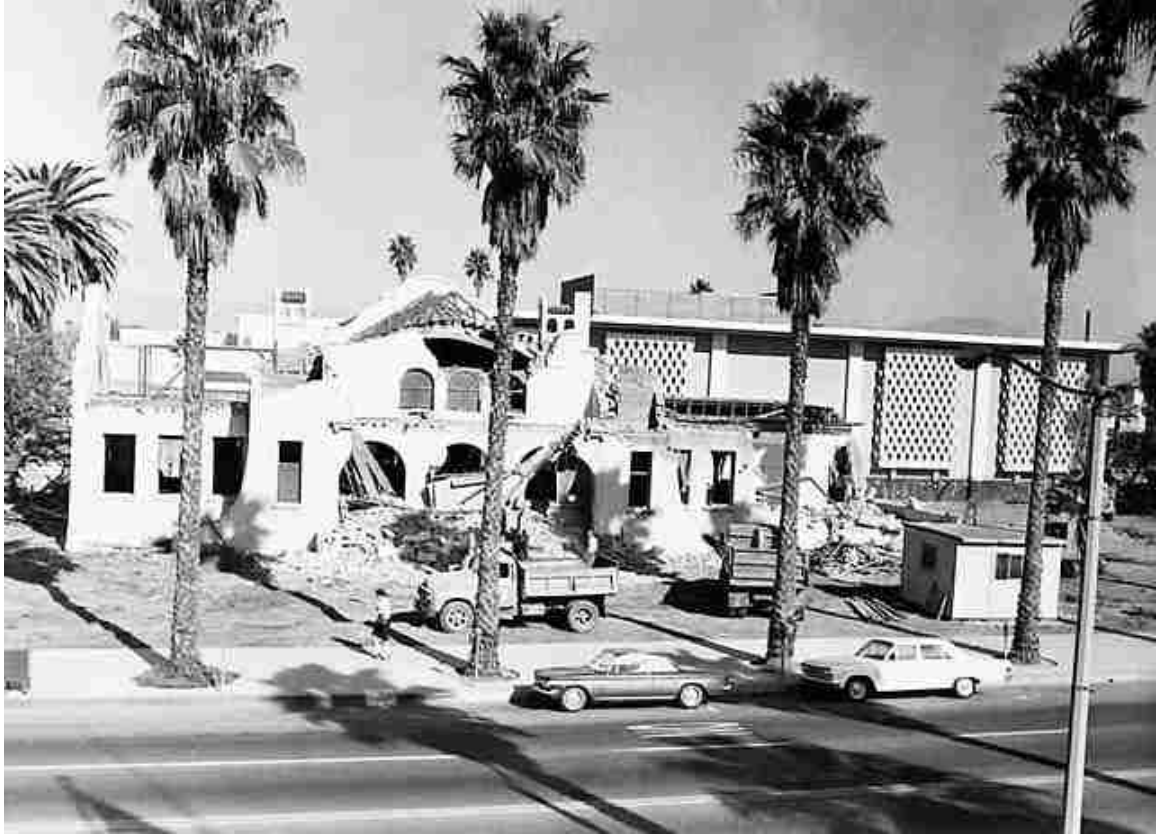
Figure 21. Demolition of Riverside's Carnegie Library in 1964, with the new library (and current Downtown Library branch) in the background. (Riverside Public Library, LIB RIV CEN CAR XIII 61 CLD2-212).
