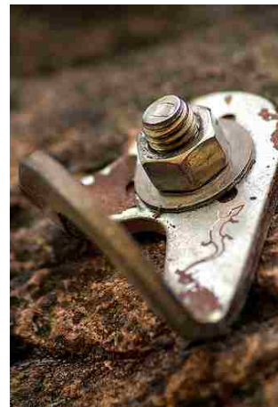
Figure 8. Bolt and bolt hanger.
