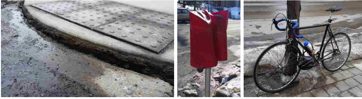
Figure 6.13: Changes to the environment not modeled by the system. (Left) winter conditions raised the curb cut out by 8cm. (Center) a parking meter covered by a bag. (Right) A bike chained to a tree.
