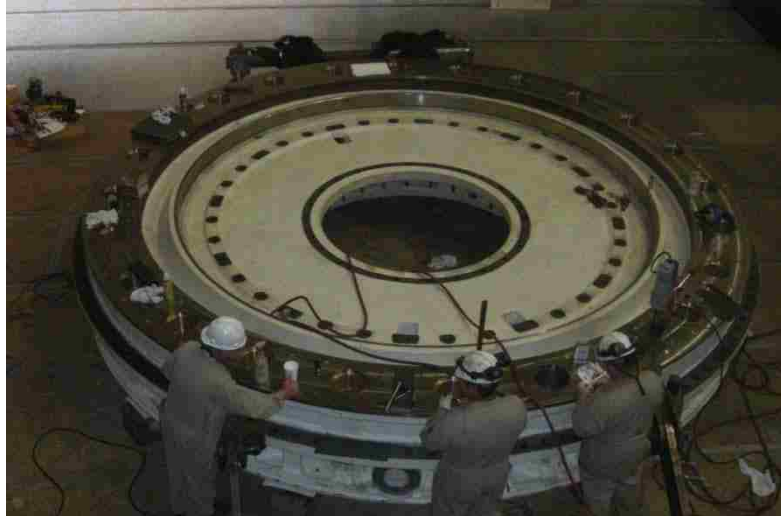
Figure 12: Hydro-Electric Mechanics (HEM's) working on the wear plates that are attached to the units head cover [2].
