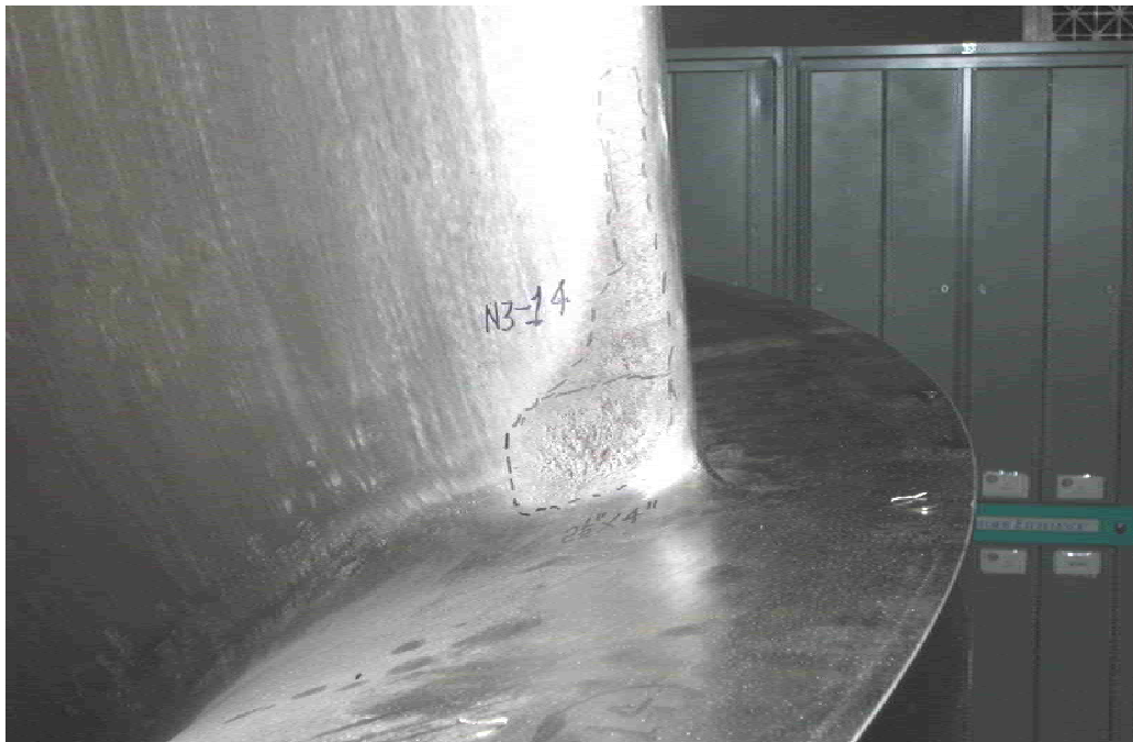
Figure 37: Erosion caused by cavitation seen on the turbine runner bucket [25].
