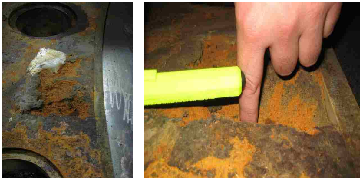
Figure 21: Damaged and Corroded wear plates [2].
