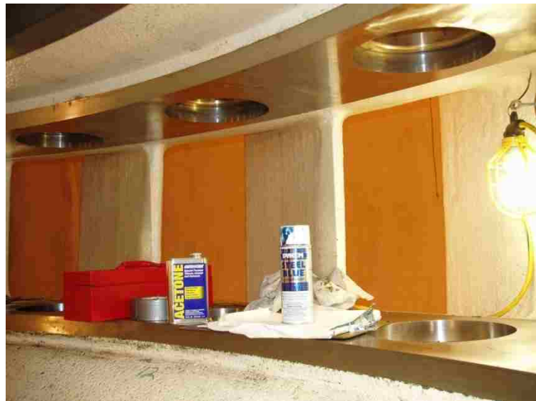
Figure 13: New wear plates installed at top and bottom of the turbine pit [2].
