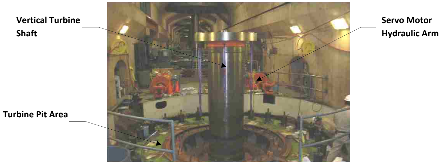
Figure 35: Turbine Pit Area, without the Wicket Gate Shift Ring [2].
