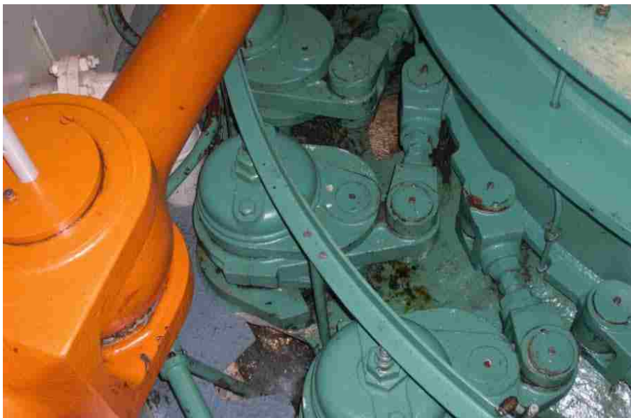
Figure 32: Wicket Gate Servo Motor Arm and Wicket Gate Mechanism [2].
