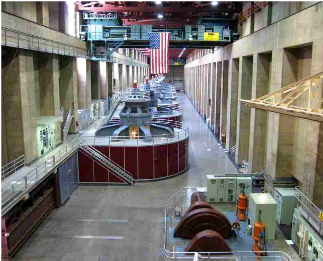
Figure 9: Hoover Power Plant, Nevada Wing [2].
