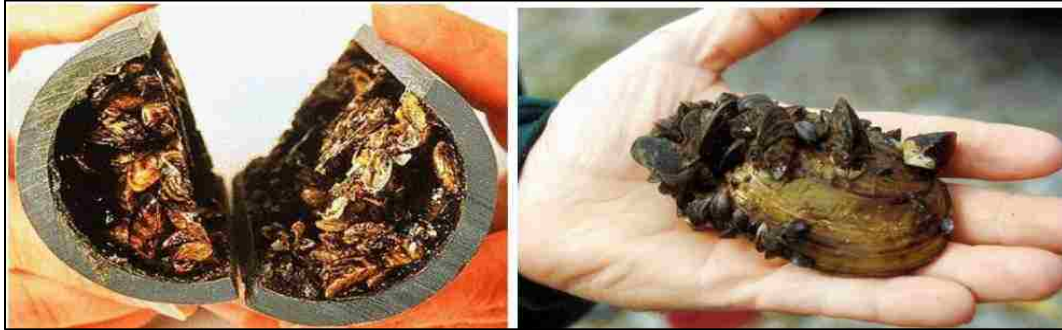
Left: Zebra mussels clogging a pipe (1,2). Right: Smaller Zebra mussels attached to larger, native mussel (1,2)
