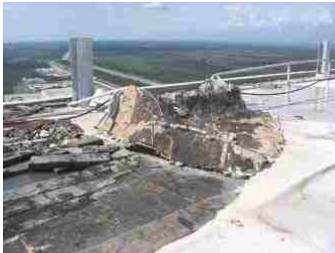
Figure 5-1 - Image of Roof Damage Caused by Hurricane (Image from John F. Kennedy Space Center Damage Evaluations)
