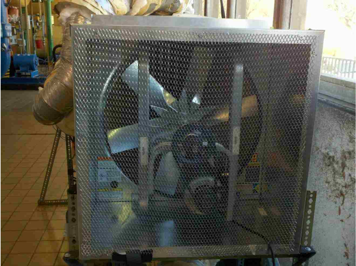
Figure 3.9 - Cooling air fan at the exit of the duct.
