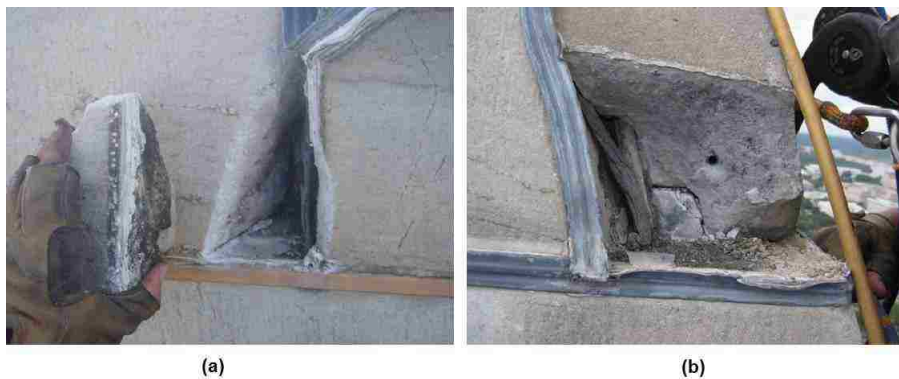
Figure 5.4. Spalling of pyramidion panels of the Washington Monument: (a) North face, (b) Northeast corner (Wiss, Janney, Elstner Associates, Inc., 2011)
