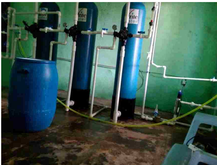
Figure 3.15. 500 LPH HAIX-NanoZr system installed at Moparlapalli by Rite Water.
