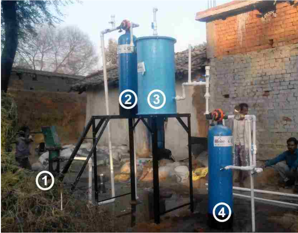
Figure 7.3. Original HAIX-NanoZr installation by Rite Water in Nuapada, Odisha. Note from Left-Right: 1) Handpump; 2) Column 1 (WAC resin); 3) storage tank/passive decarbonator; 4) HAIX-NanoZr.
