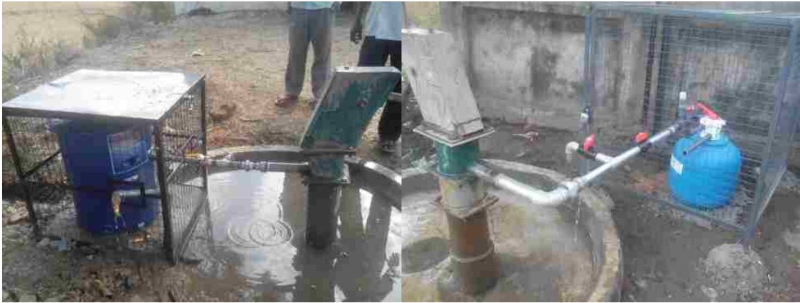
Figure 7.5. Fluoride removal systems from HES (L, OxiMax) and Ion Exchange (R, Indion-RS-F). Note the much smaller volume of HES and Indion systems.
