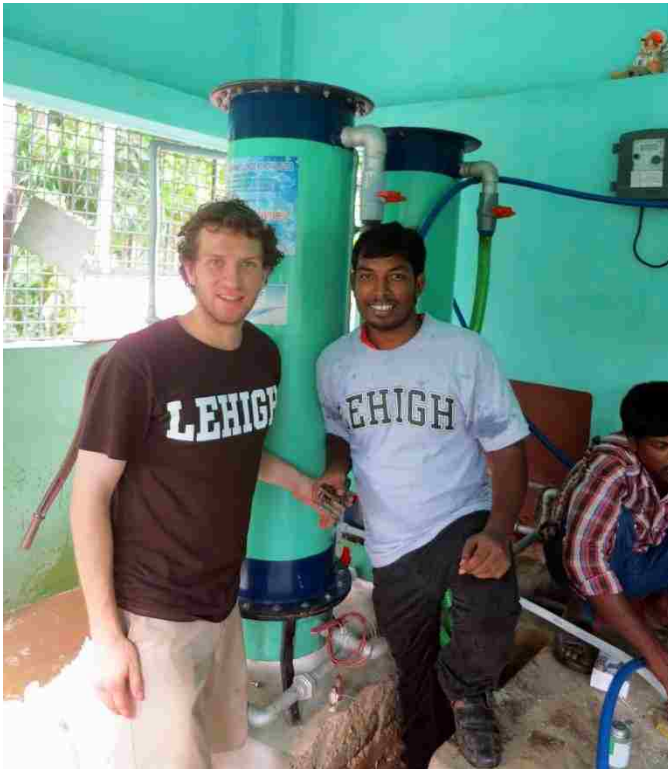
Figure 5.7. Anil Shaw and Mike German installing an SAC-Fe system in Binimaypara (N. 24 Parganas, West Bengal); a technician from Ramkrishna Water Mission is partially off-screen.
