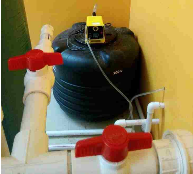
Figure 3.13. Close-up of 200 L chemical dosing tank behind Column I with chemical-resistant pump at the Baduria treatment system.
