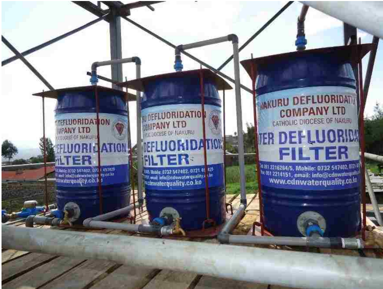
Figure 11.7. HAP filters installed by JB Drilling in a treatment system outside Nakuru.
