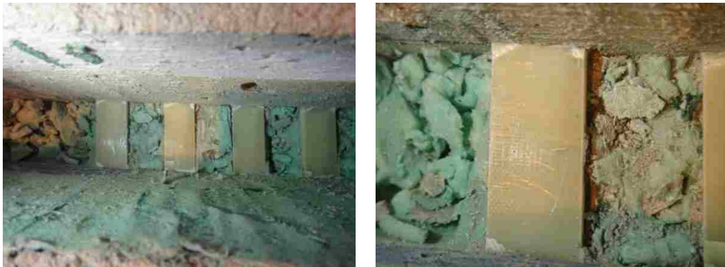
Figure 70: Post-failure examination of exposed shear tie legs
