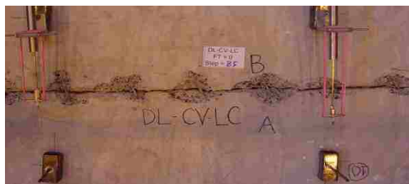
Figure 4.29. Damage state at 1.0-in shear opening
