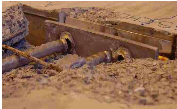
Figure 4.40. Damage state at 2.15-in shear opening
