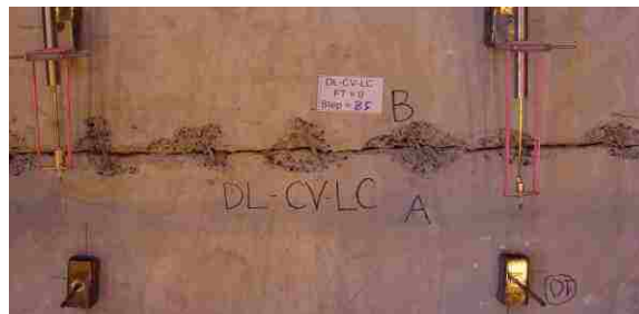
Figure 4.26. Damage state at 0.77-in shear opening
