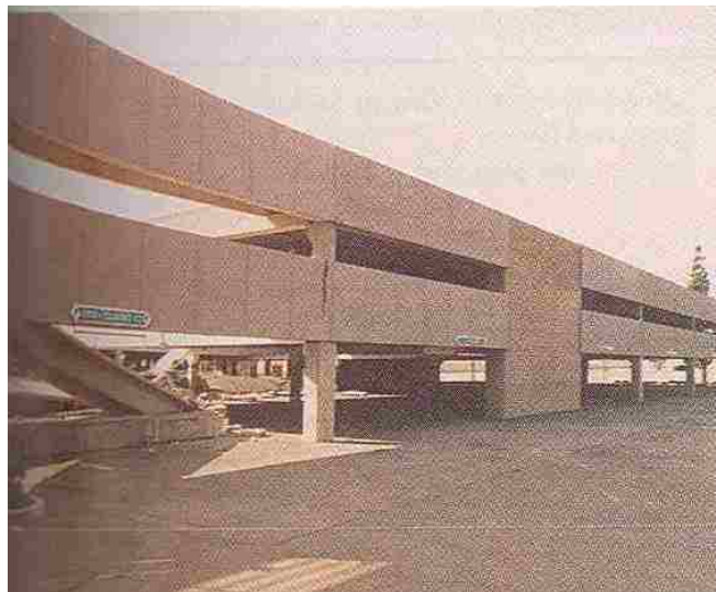
Figure 2.18. Precast panels collapsed and structural walls remained intact
