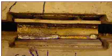
Figure 4.18. Damage state at 0.5-in tensile opening
