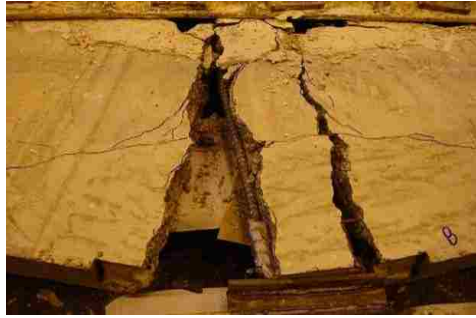
Figure 4.15. Damage state at 5.0-in tensile opening
