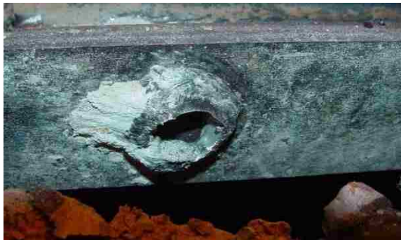
Figure 4.34. Damage state at 3.5-in shear opening
