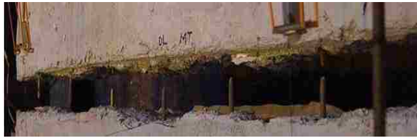
Figure 4.10. Damage state at 2.5-in tensile opening
