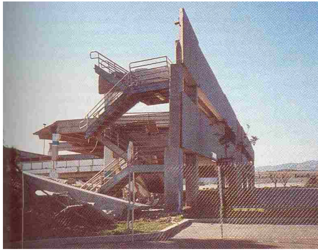
Figure 2.17. Collapsed parking garage (Iverson and Hawkins 1994)
