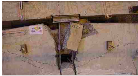
Figure 4.19. Damage state at 2.0-in tensile opening
