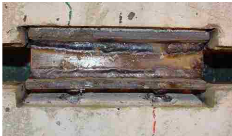
Figure 4.16. Damage state at 0.39-in tensile opening
