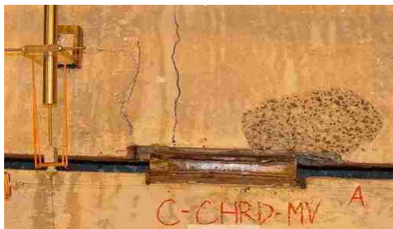
Figure 4.32. Damage state at 0.75-in shear opening
