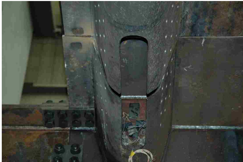
Figure 112 Lack of alignment of the ribs
