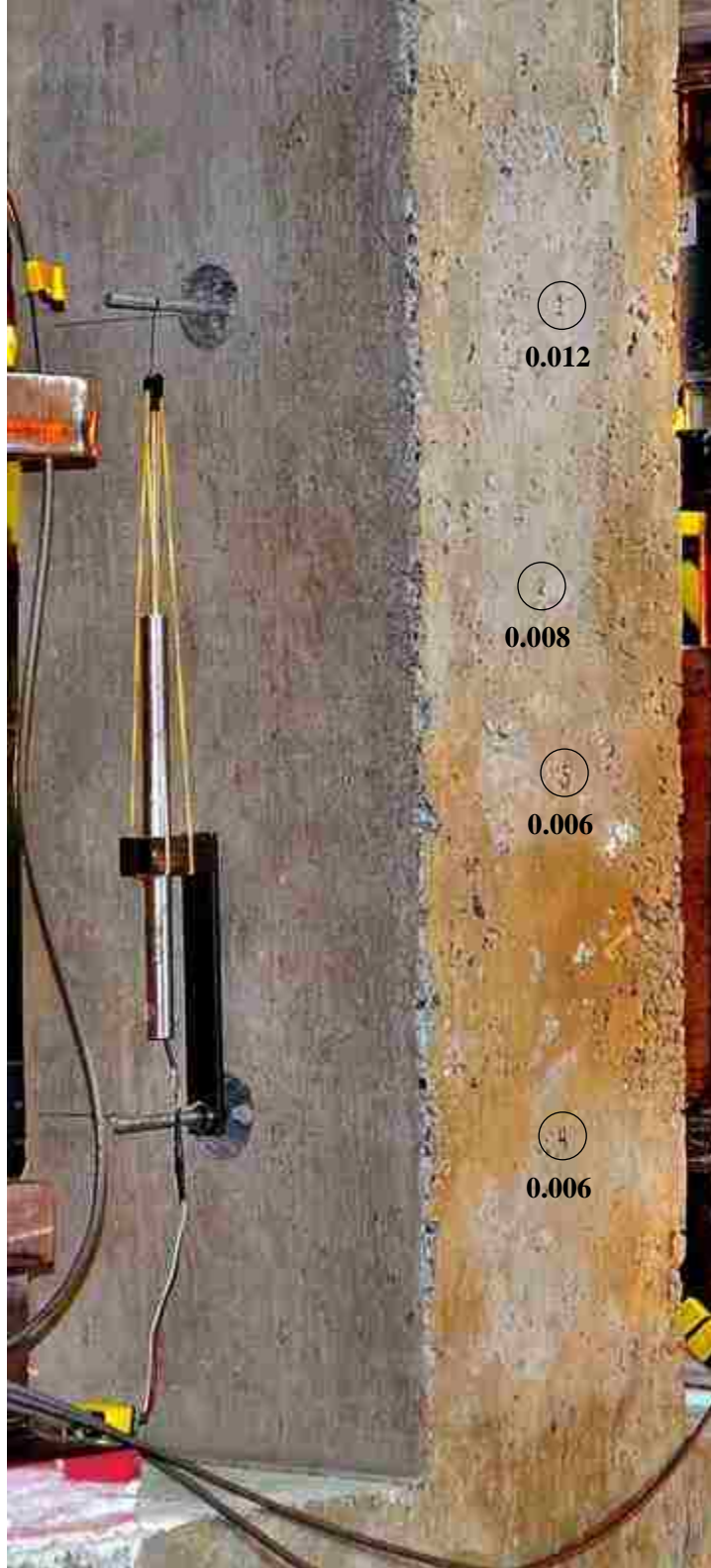
Figure 4-92: Cracks on west face of TS02 at Load Step 09
