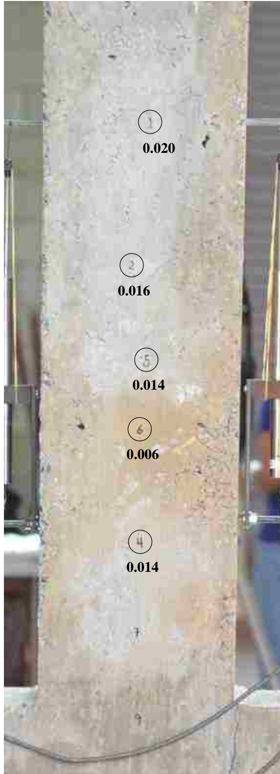
Figure 4-94: Cracks on east face of TS02 at Load Step 15
