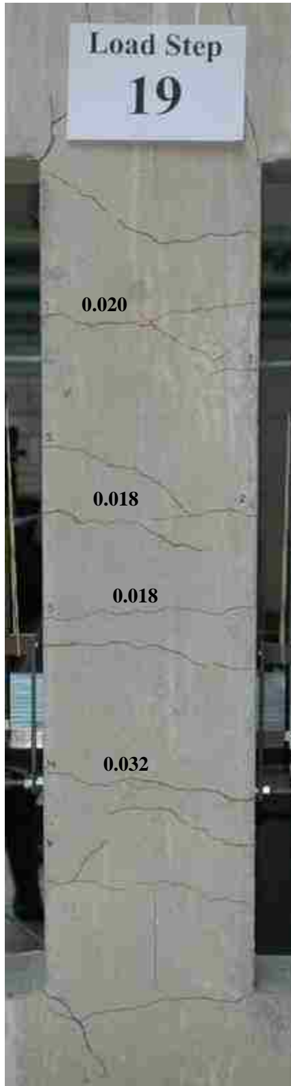
Figure 4-97: Cracks on west face of TS02 at Load Step 19
