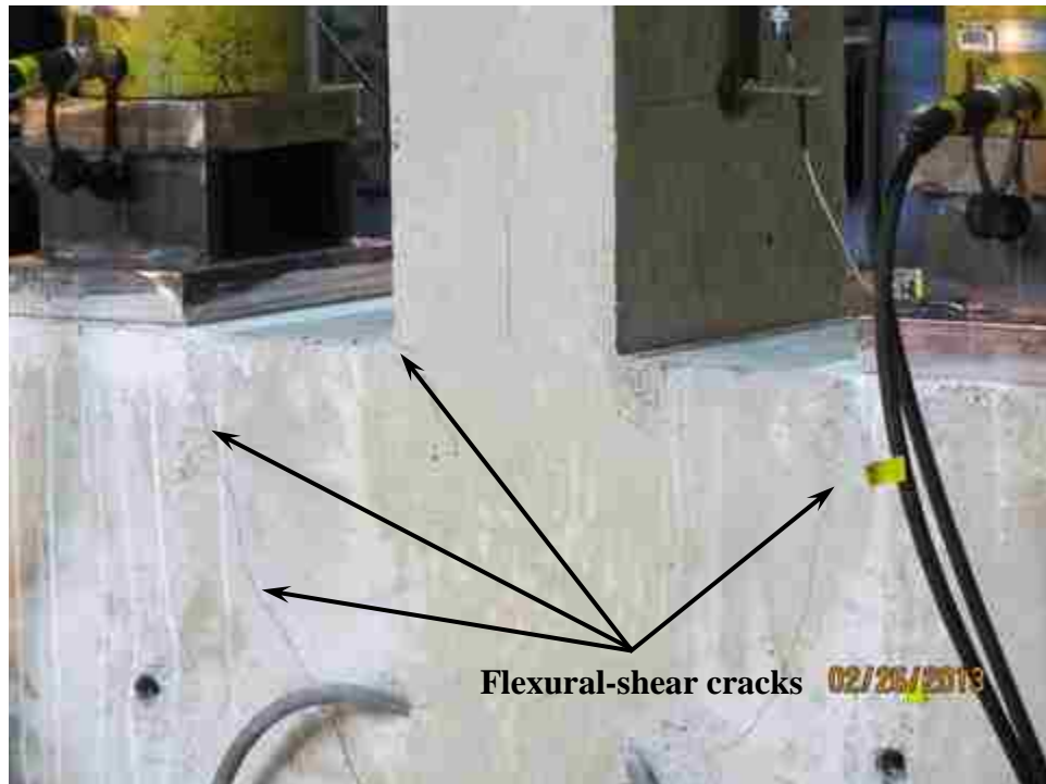
Figure 4-89: Flexural-shear cracks in bottom beam of TS02
