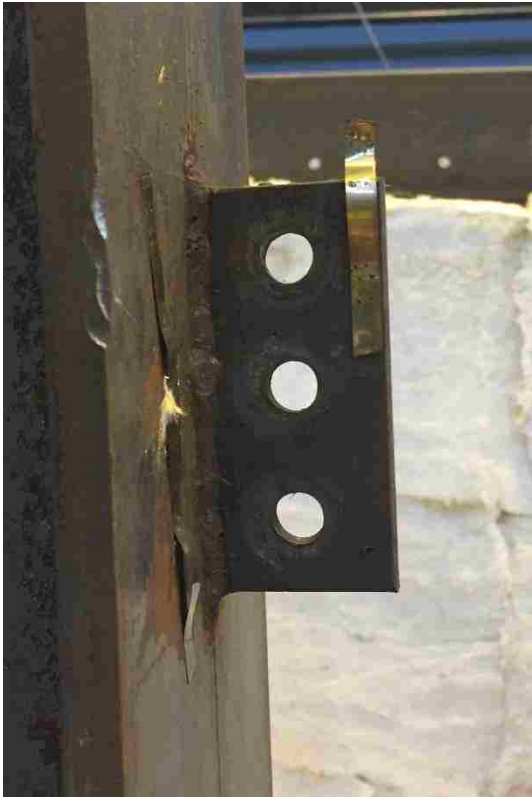
Figure 13 – Shear tab connection after the test
