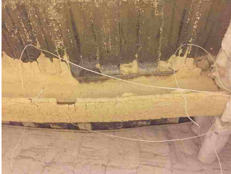
Figure 52 – SFRM chunks missing on flanges
