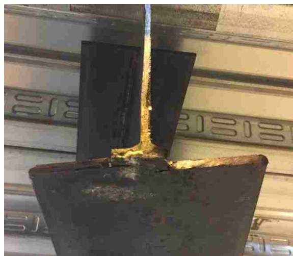
Figure 74 – Rupture in Web to Flange Connection
