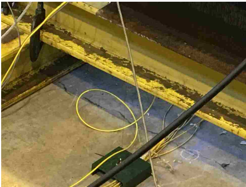
Figure 11 – Close up of longitudinal crack
