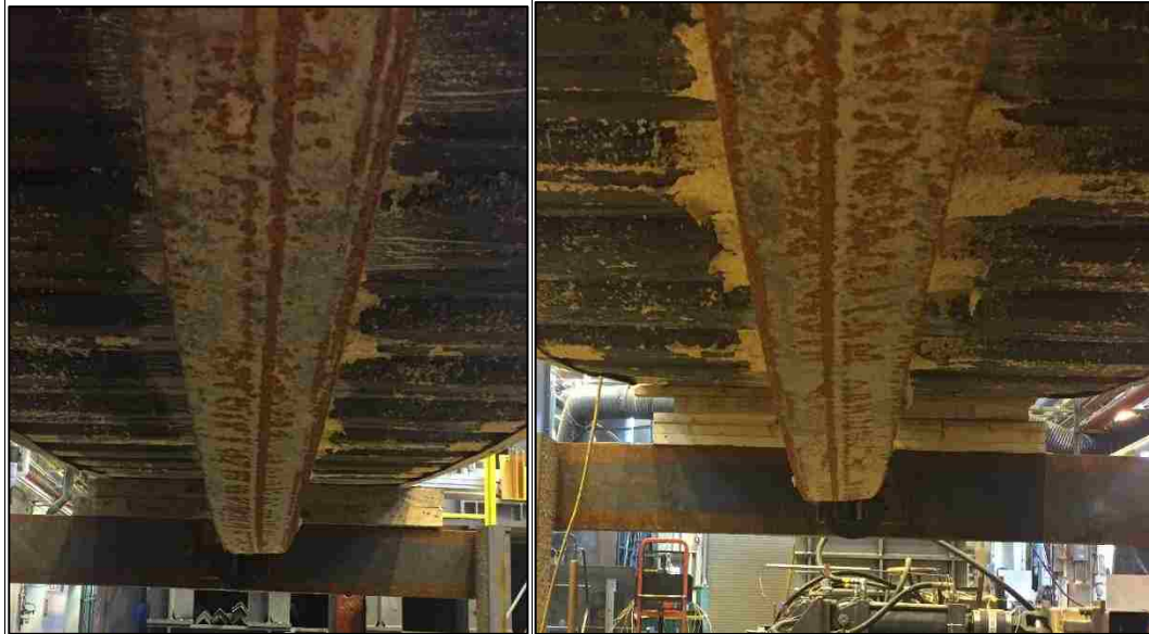
Figure 54 – Test 3 Beam Twist at Failure
