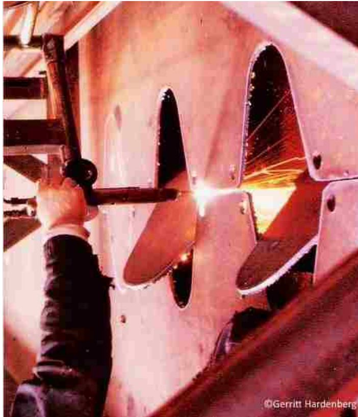
Figure 27 Burning of rib profiles in floor beam web (reproduced from Gerritt Hardenberg)
