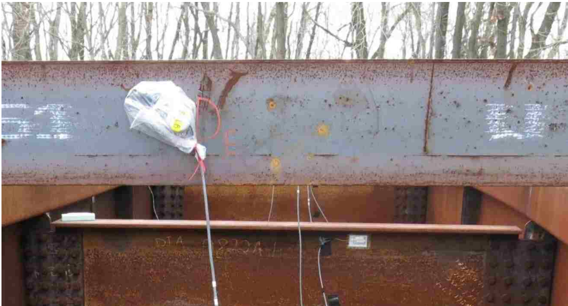
(c) Inclinometer attached to loading beam to measure rotation in parallel plane
