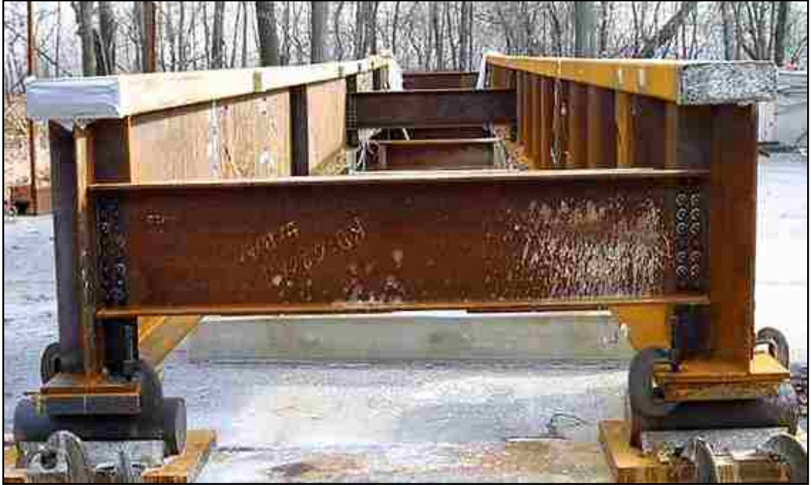
Figure 2.1 Straight TFGs with concrete-filled rectangular steel tube top flange (Wimer and Sause, 2004)
