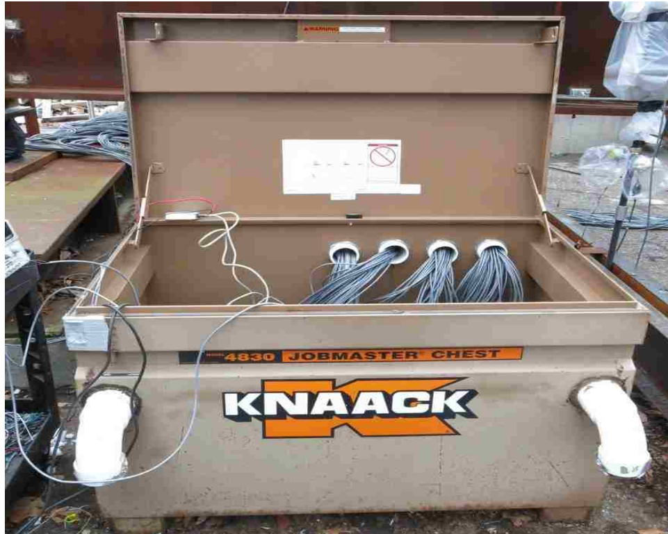
(a) Protective metal box
