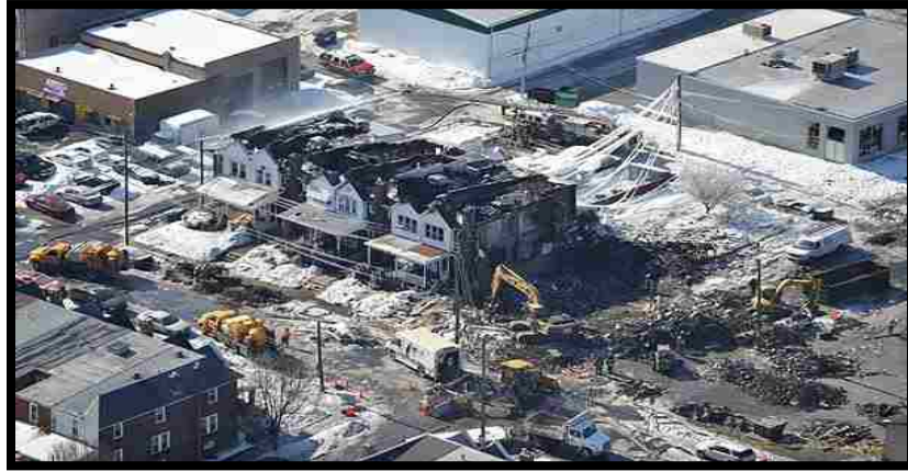
Figure 17 Allentown's natural gas explosion [3].
