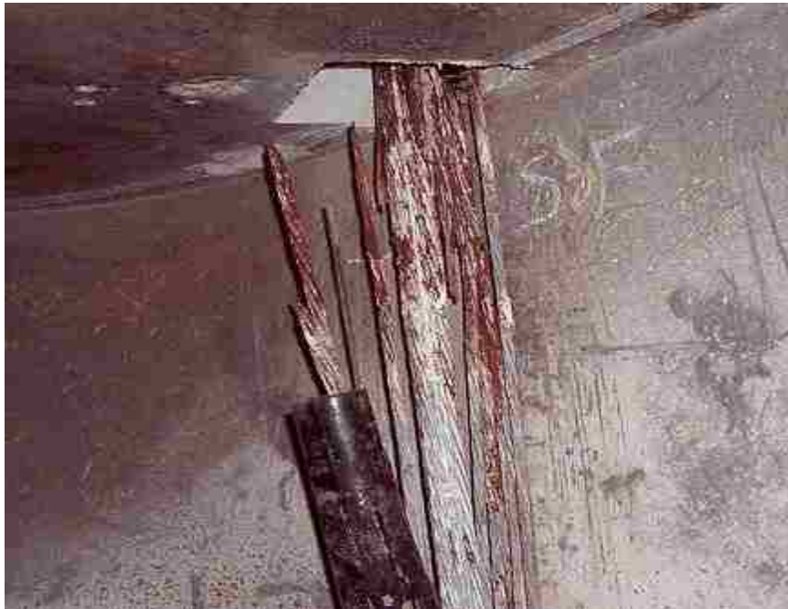
Figure 2.2 - Corroded tendon in the Sunshine Skyway Bridge (FDOT, 2002).
