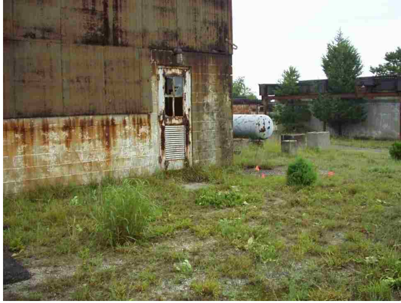
Figure 4. Outside the restroom facility. Notice the concrete apron and the orange flags designating areas of elevated activity
