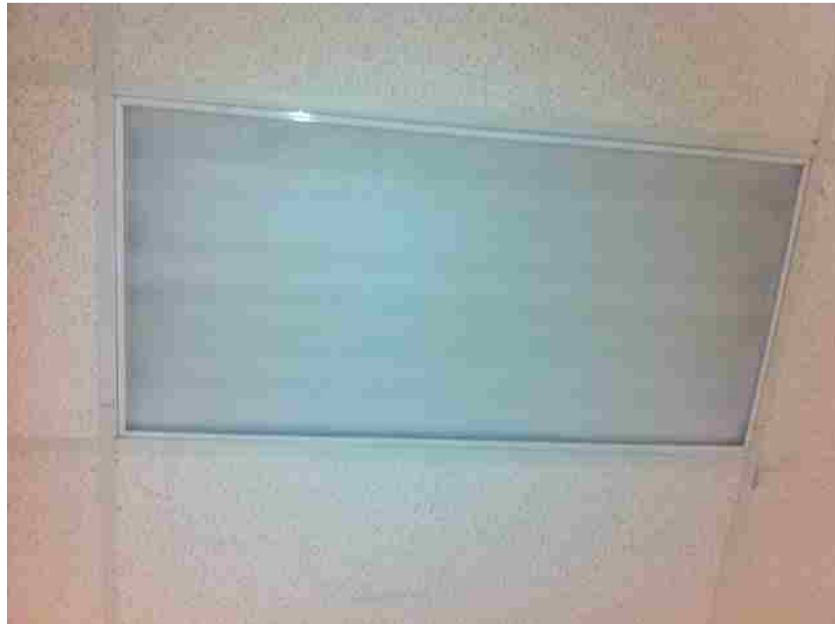
Figure 3.22 The fluorescent ceiling fixture used in this study
