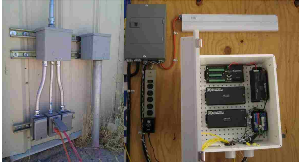
Figure 10 - Electrical and Data Logging Components
