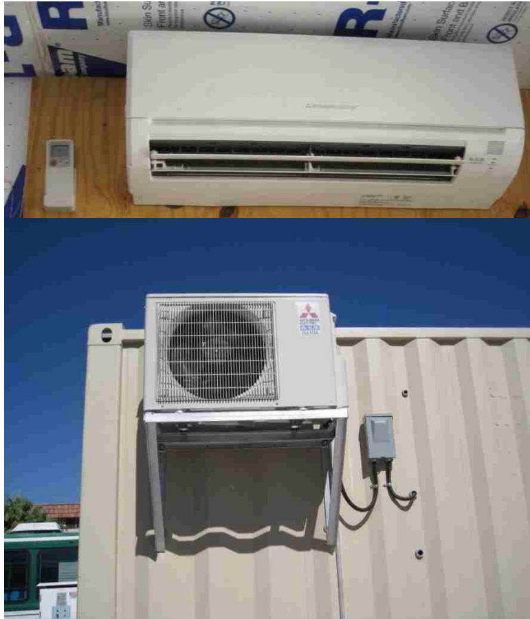
Figure 11 - Mini Split Ductless A/C System
