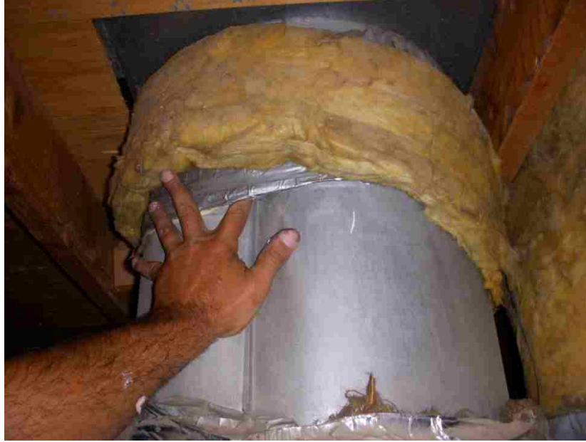
Figure 22. Gap located on the outer surface of duct located in the attic of house # 8
