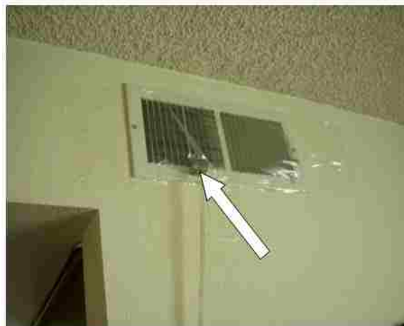
Figure 11. Pressure probe installed on the register grill
