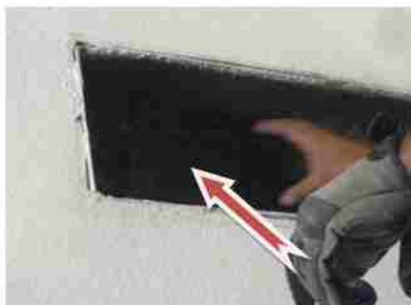
Figure 17. Obstruction shield installed to improve air flow distribution in house #5
