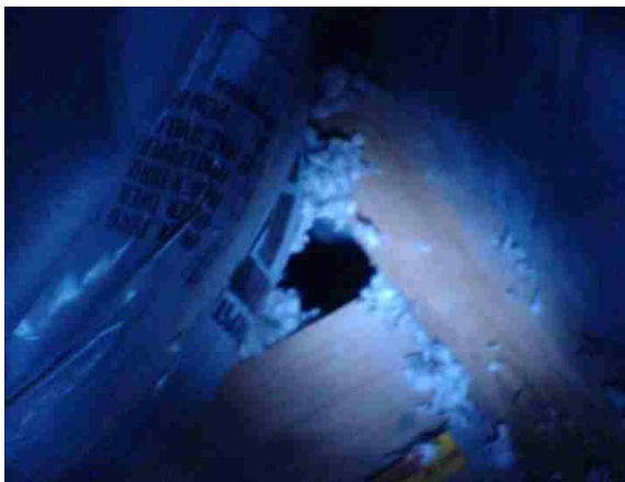
Figure 14. Hole inside the insulation of the attic of house #5
