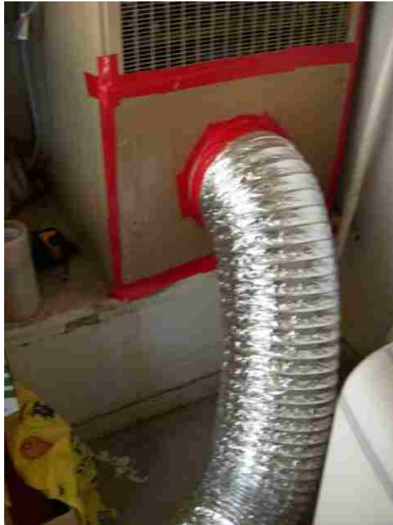
Figure 9. Duct Blaster installed in system to perform duct pressurization test
