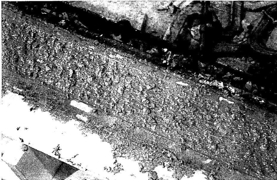
Figure 7-7: As-Placed Surface Finish
