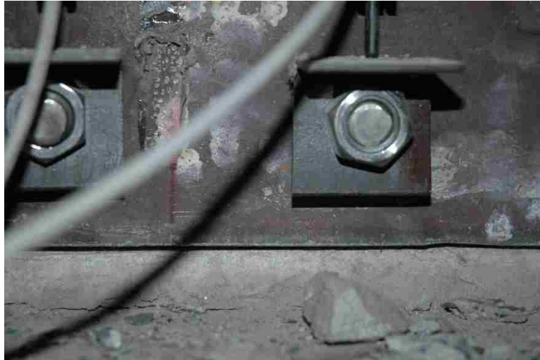
Figure 5-12 - Lack of Damage at Bottom Corner of Panel - East Side
