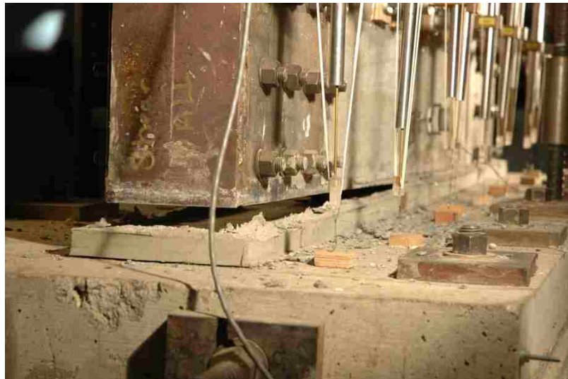
Figure 5-7 - Gap Opening at 1.5% Roof Drift (Eastward Loading)
