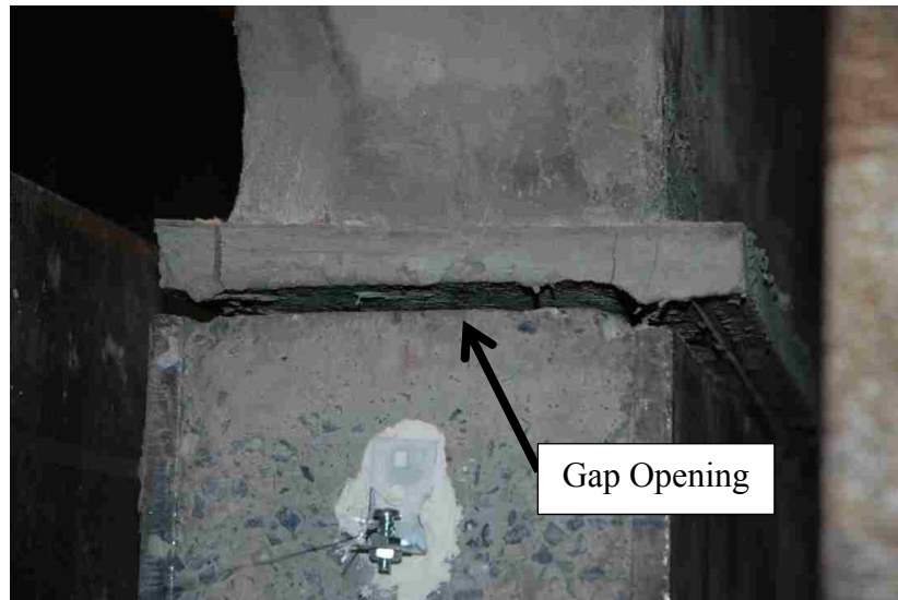
Figure 5-24 - Gap Opening at Joint between First and Second Panels 2% Roof Drift (Westward Loading)
