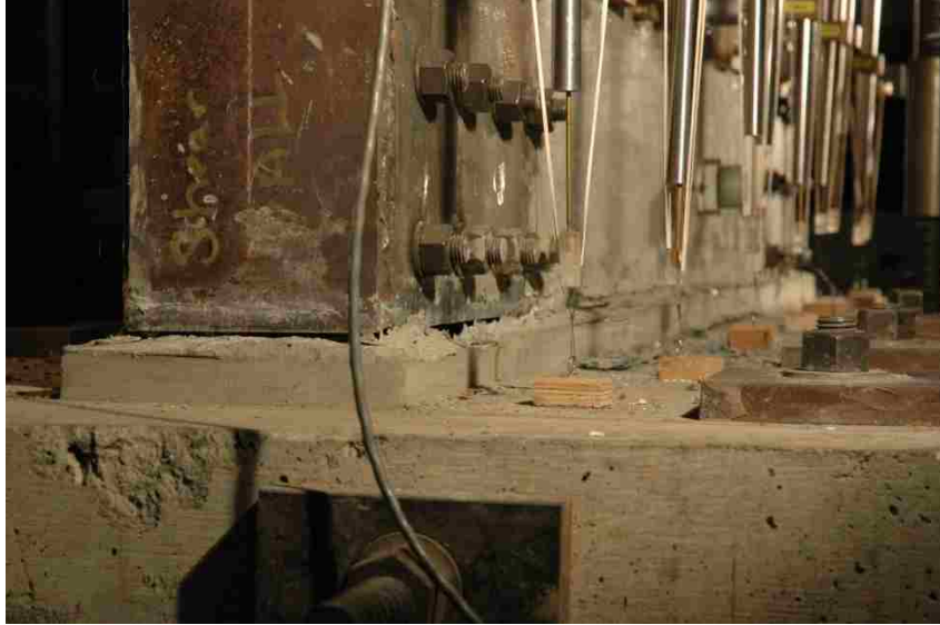
Figure 5-5 - Gap Opening at 0.75% Roof Drift (Eastward Loading)
