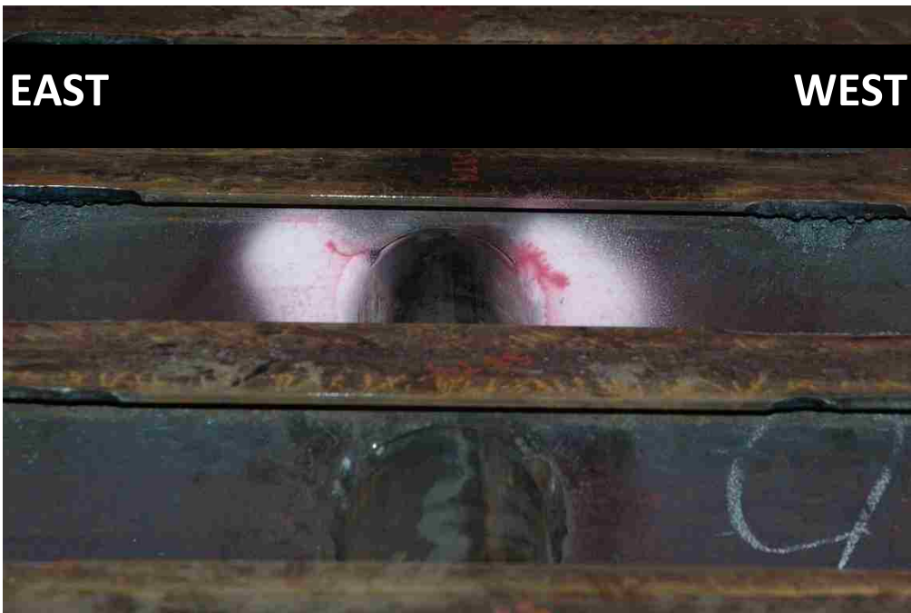
Figure 63. Specimen #1, cracks at S9-T4 intersection, shown with dye penetrant
