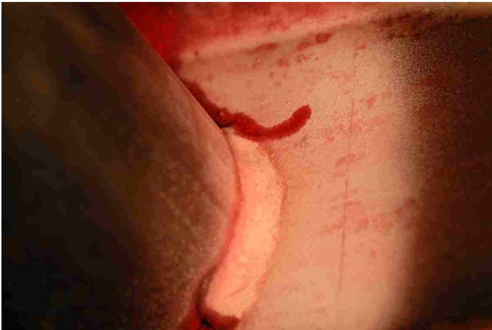
Figure 65. Specimen #2, crack at west weld of the S9-T1 intersection
