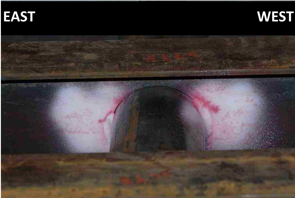
Figure 62. Specimen #1, cracks at S7-T3 intersection, shown with dye penetrant
