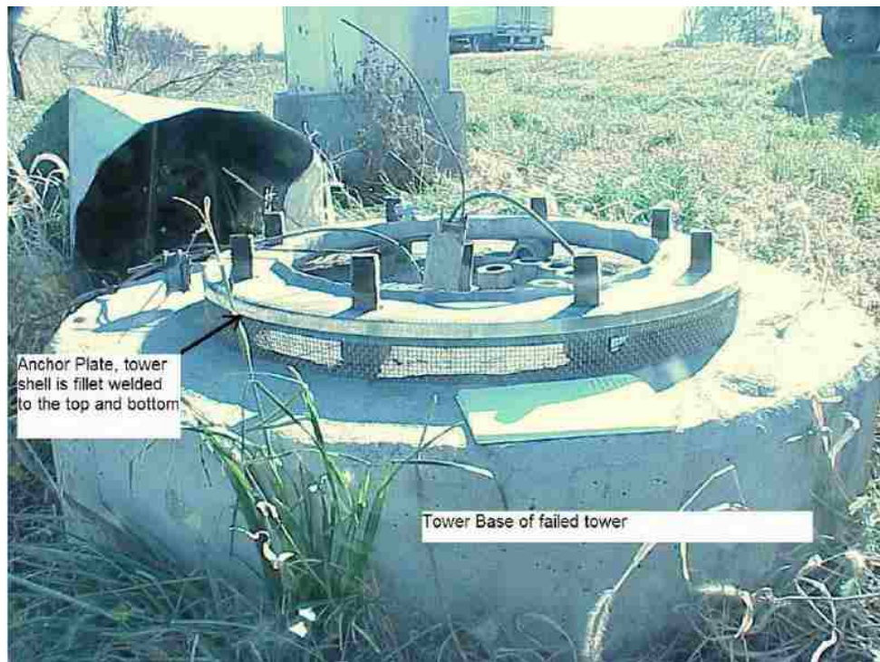
Figure 4. Close-up of collapsed tower ( reprinted from Dexter, 2004 )
