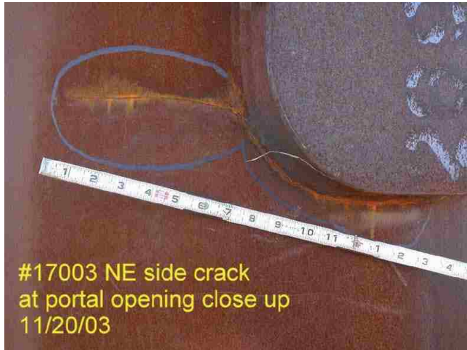
Figure 5. Handhole crack at corner ( reprinted from Koob, 2006 )
