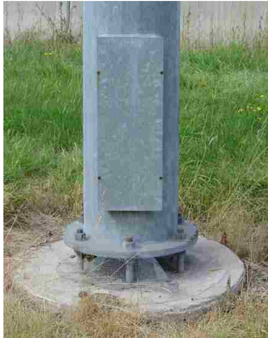
Figure 3. Example of a handhole on an in-service structure
