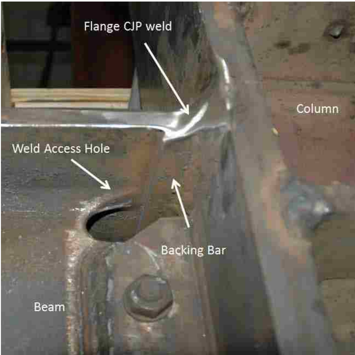
Figure 4.21- Ground Floor Top Flange with Run Off Tabs Removed and Weld Ground
