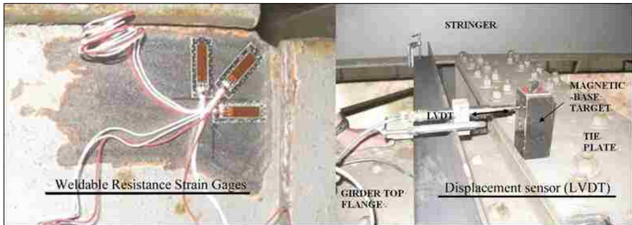
Figure 2-6: Sensors placed on critical locations of the bridge
