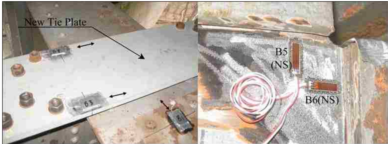
Figure 2-9: Strain gages installed on the tie plate (B3, B4), on the top flange of the girder (B1) and on the cantilever bracket web (B5, B6)
