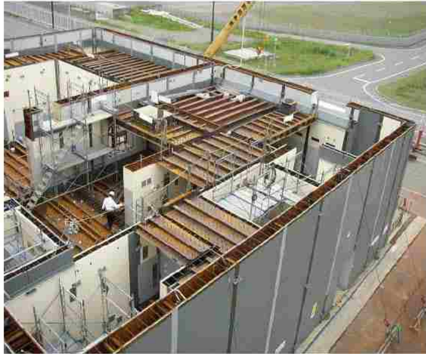
Figure 4.1: Steel Concrete Composite wall structure under construction phase (International Atomic Energy Agency)
